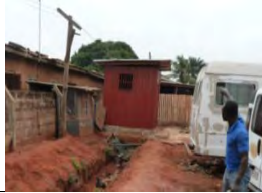
B. Trench routed under structure? OR structure rebuilt after temporary relocation? OR new structure built over trench
