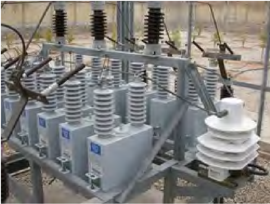
FIGURE 12 Typical capacitor installation at substation
