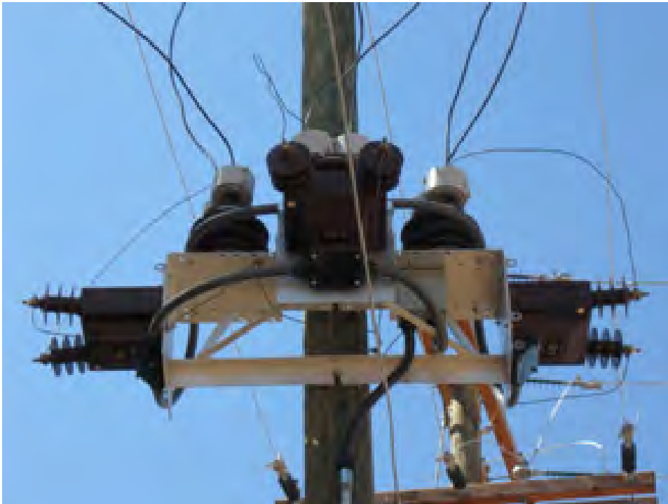
FIGURE 7 MV PT and CT metering cluster on pole
