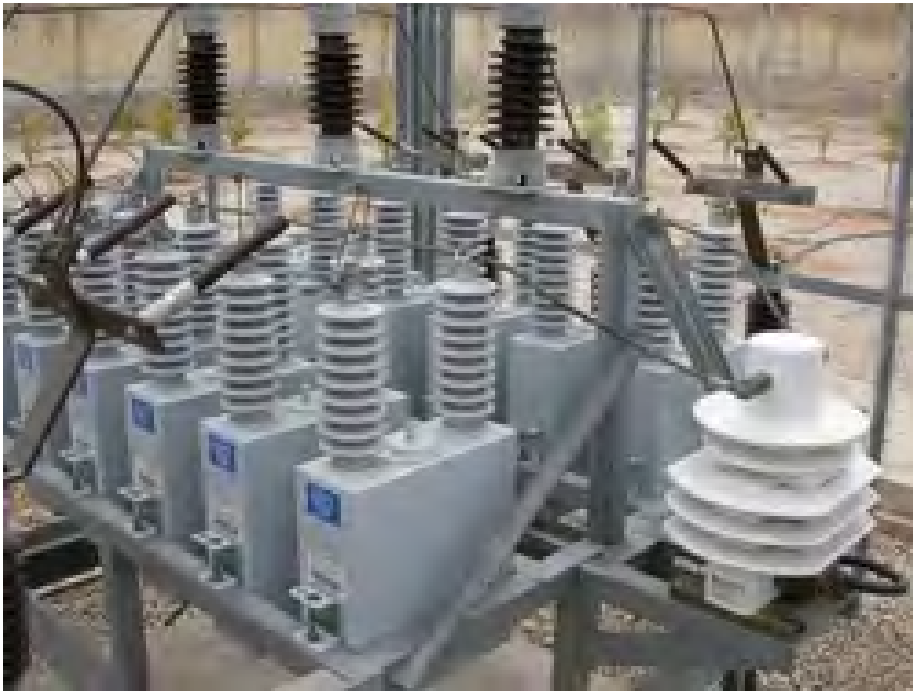
FIGURE 12 Typical capacitor installation at substation
