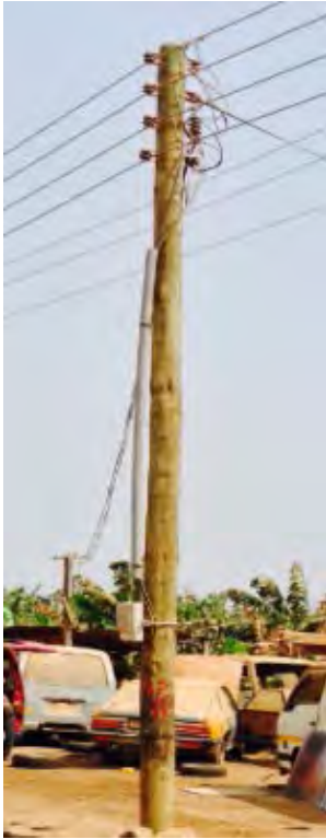
FIGURE 6-5 Typical LV Distribution Line
