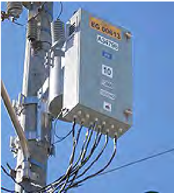
FIGURE 2 Meter box mounted on the pole with din rail style meter. All the wires coming out of the box are already metered.
