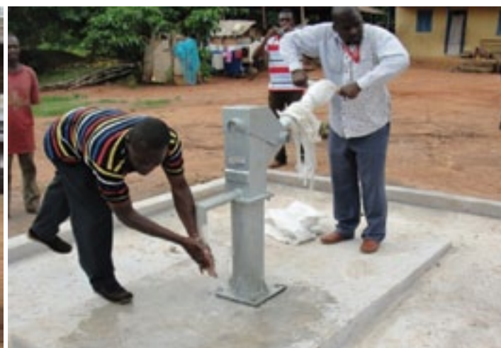
A Borehole with hand-pump at Tadieso in the Afram Basin Zone.
