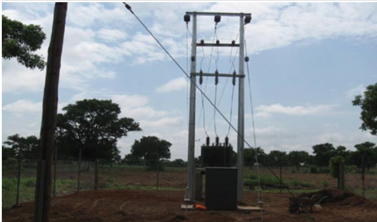
A 315kVA/ 34.5/0.415kV PMT Transformer installed at the Integrated Tamale Food Company (ITFC) in the Savelugu Nanton District of the NAZ.
