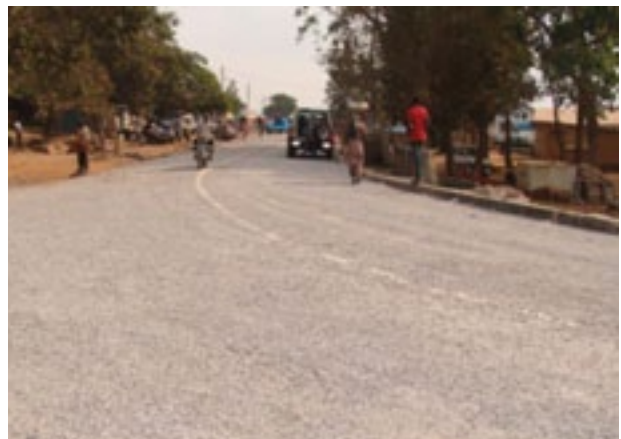
A section of the Agogo-Afrisere Trunk Road through Agogo township after construction
