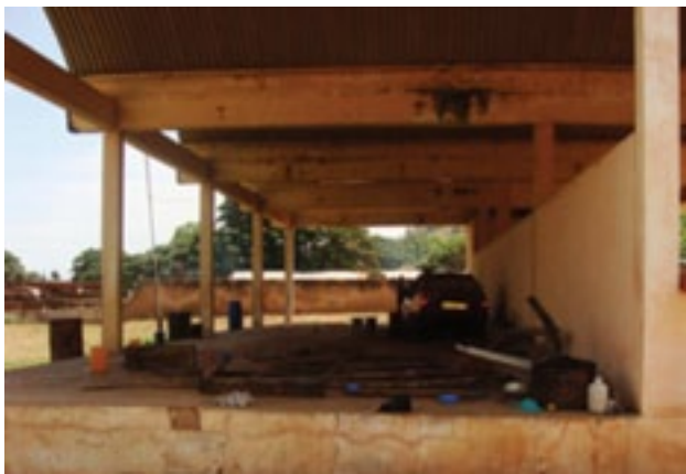
Partial view of the Ferry Terminal at the Adawso end before construction
