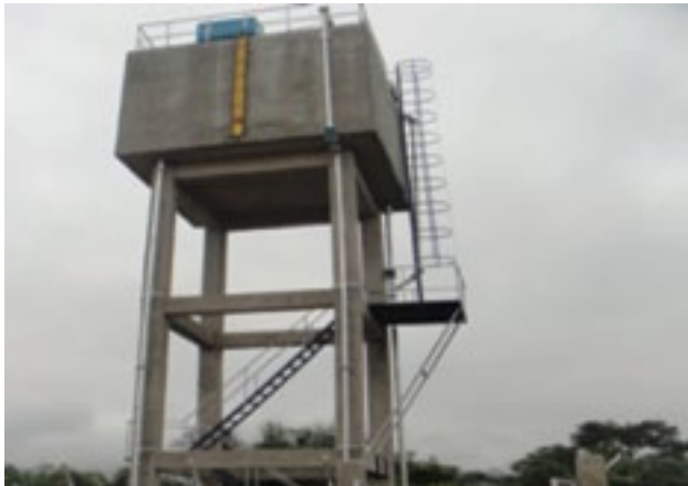
50 m3 High level tank at Yonso in the Mampong Municipality of the Afram Basin Zone
