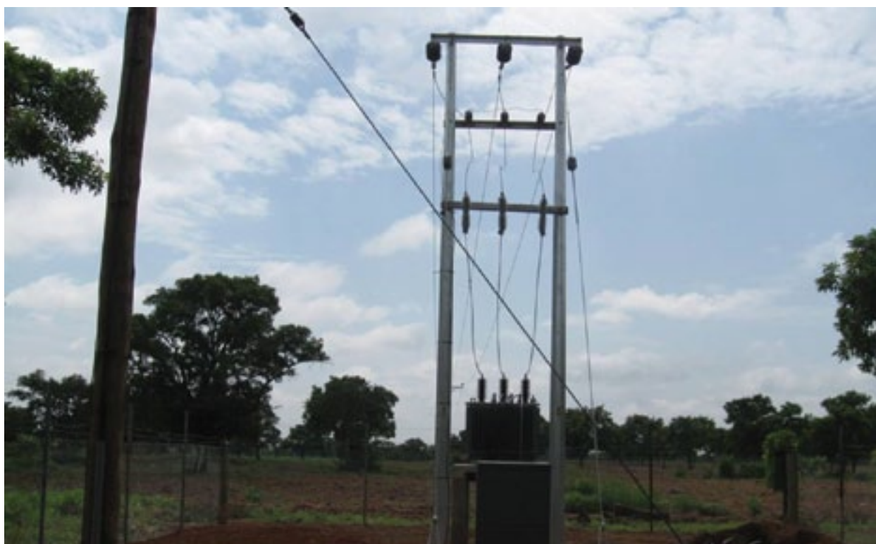
A 315 kVA, 34.5/0.415kV PMT Transformer installed for the Tamale Integrated Food Company (ITFC) at Gushie in the Savelugu Nanton District.
