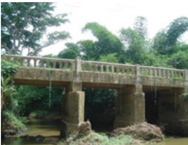
A pre-construction view of the Kwanyako Bridge along the Akoti-Desum-Kwanyako Feeder Road in the Central Region.
