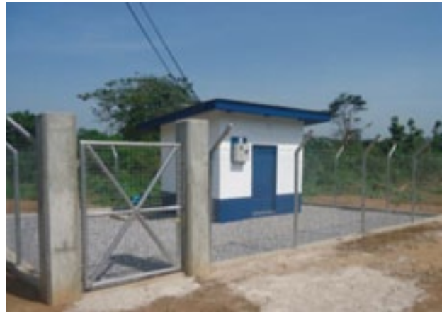
Pump house at Apaah in the Sekyere Central District of the Afram Basin Zone
