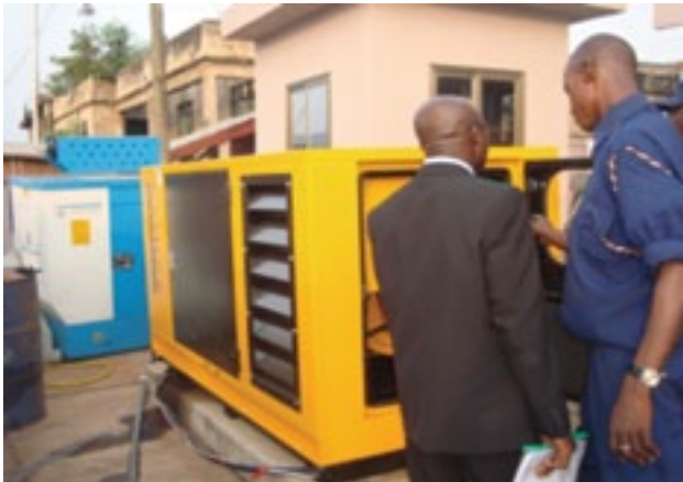
Secondary Power has been a critical component of the new computerized systems
