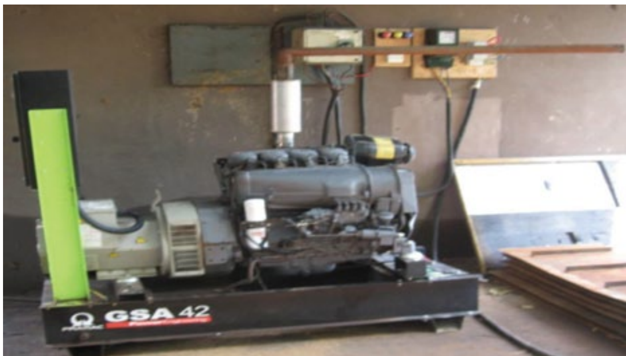
Electricity generating system used by the Tamale Integrated Food Company (ITFC) before connection to the national grid.
