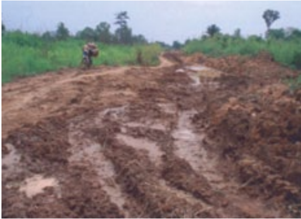
An impassable area of a section of the Agogo-Dome Trunk Road before construction
