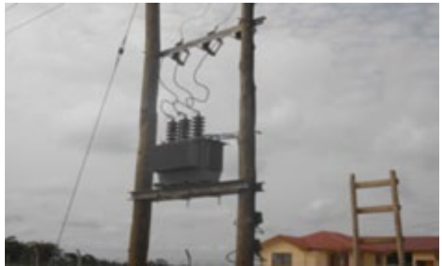
Pole mounted with a 100KVA Transformer connecting ABC Site to National Power Grid. Same was done for all ABCs.
