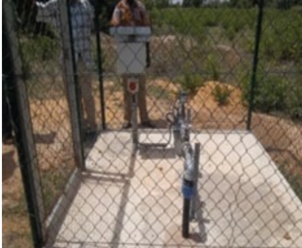
Fenced Borehole completed and well mechanized for Janga Polyclinic in the West Mamprusi District of the Northern Agricultural Zone.
