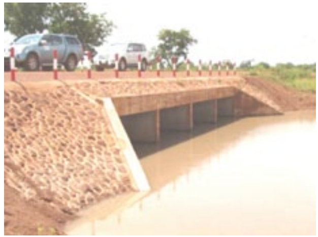
A Post-construction view of the Bridge constructed to correct the perennial flooding of a section of the Savelugu Kpandu Batoyili Feeder Road in the Northern Region.
